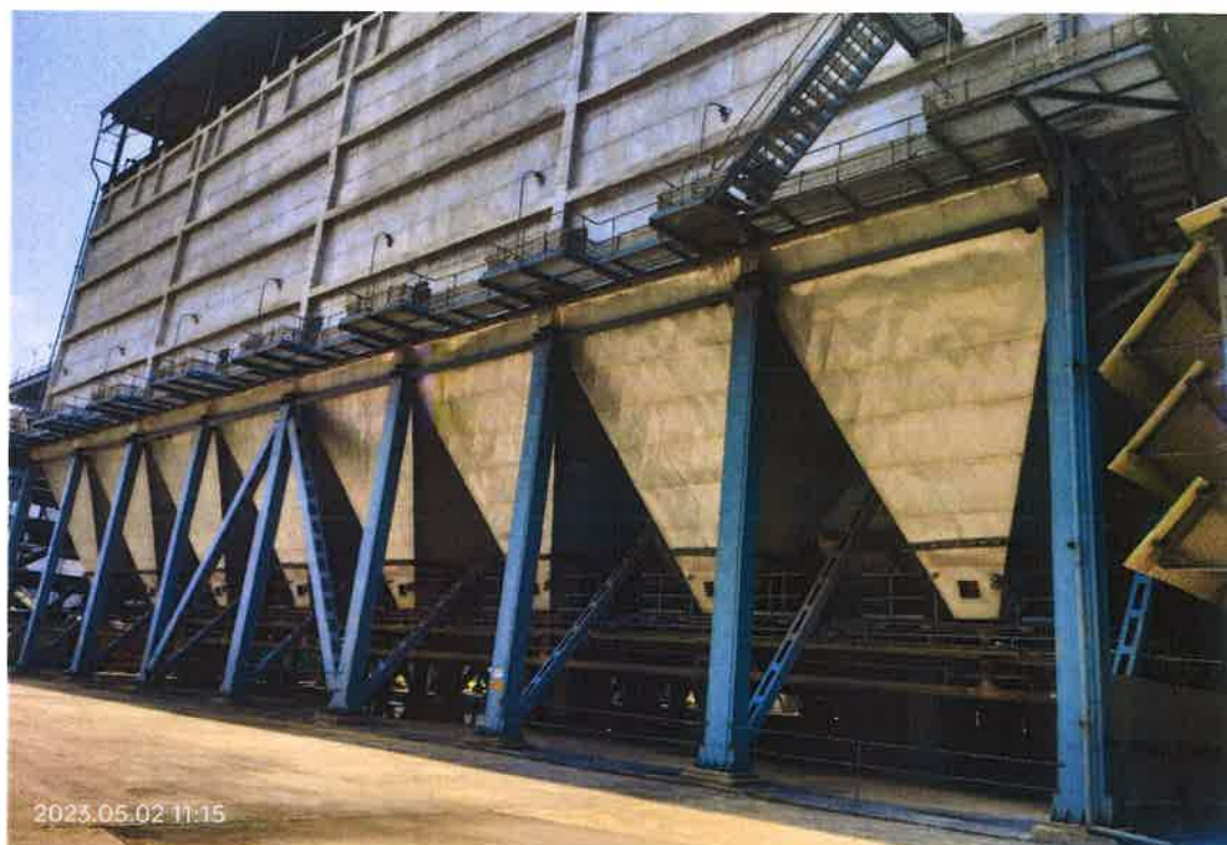
ESP installed for particulate emission control
