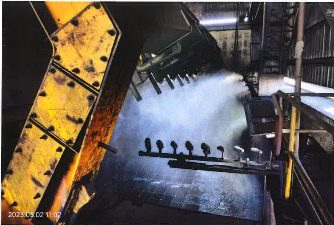
Fogging system at wagon tippler area
