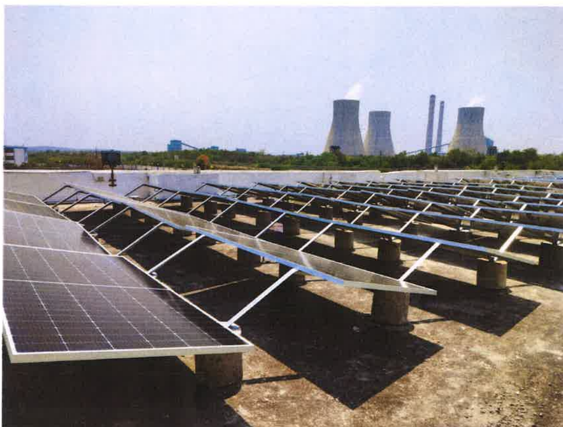
Roof Top Solar Installed at Hospital Building
