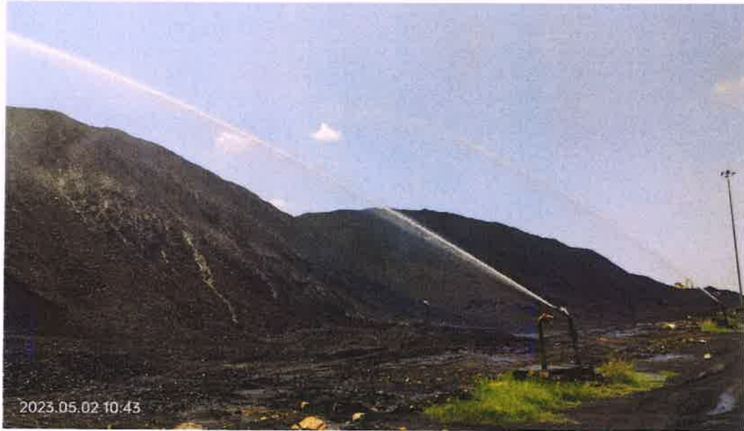
Dust suppression system installed at coal yard
