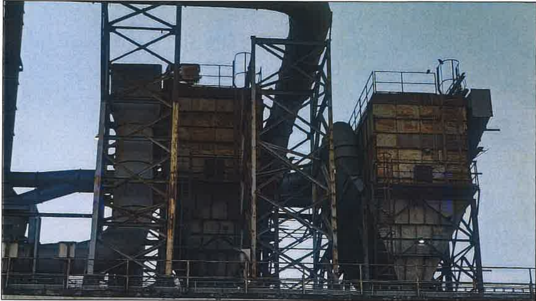
Bag filter installed for particulate emission control
