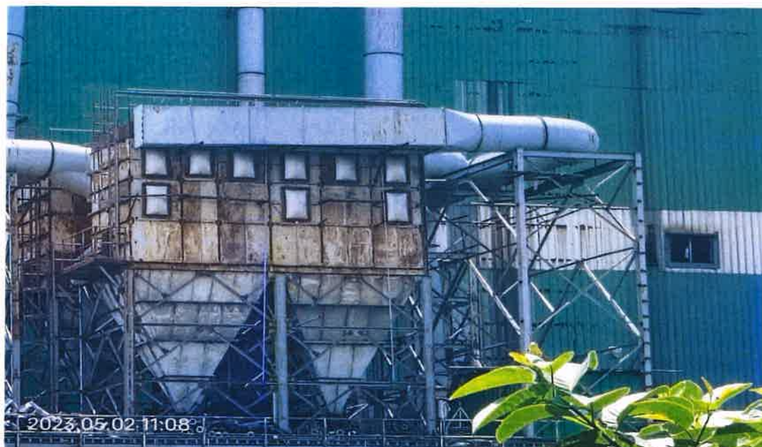
Bag filter installed for particulate emission control
